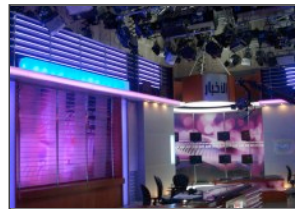
DMI invests in complete LED lighting solution for Syrian TV's new studio.
